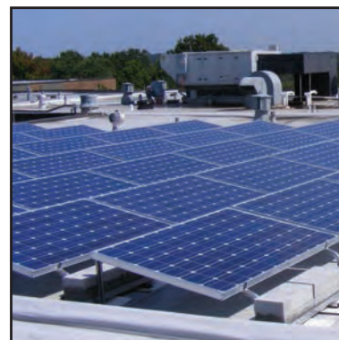
Fred W. Nimmer Place with rooftop solar panels for electric energy, 2011
